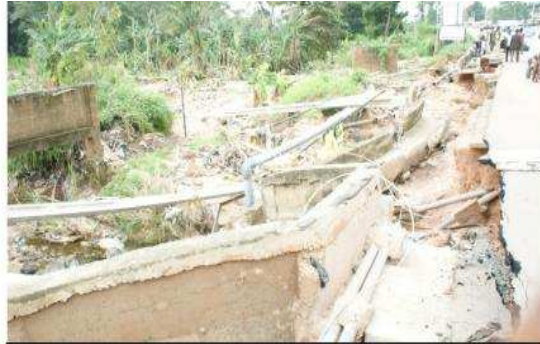
Damaged UI fence along Orogun Road
