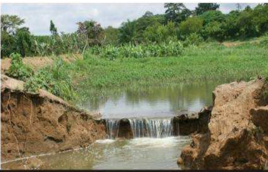
The damaged newly constructed Fish Pond
