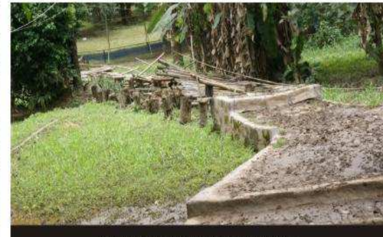
Damaged Bamboo Bridge in the Zoo
